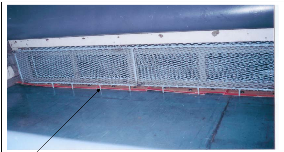
Photograph of final system after fitting the screens and laying Glue Boards inside it
